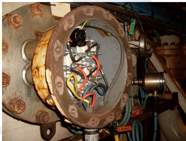
Figure 2 - Same heater as Figure 1, showing acceptable internal condition
