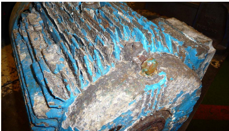
Figure 4 - Example of corrosion of aluminium motor housing
