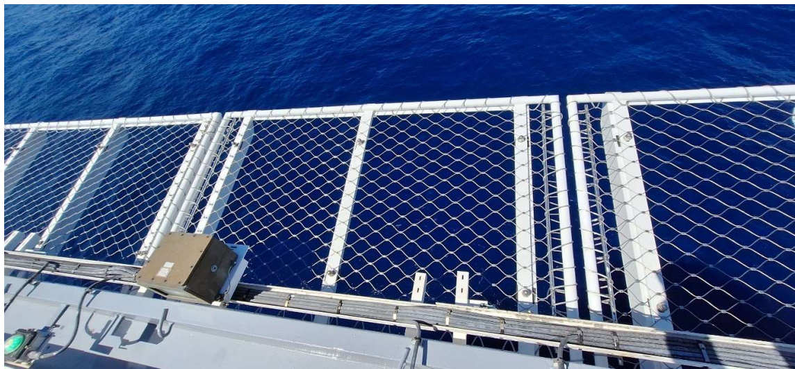
Figure 66: Steel Wire helideck Perimeter Safety Net
