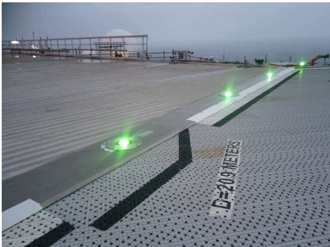
Figure 48: Helideck Perimeter Lights
