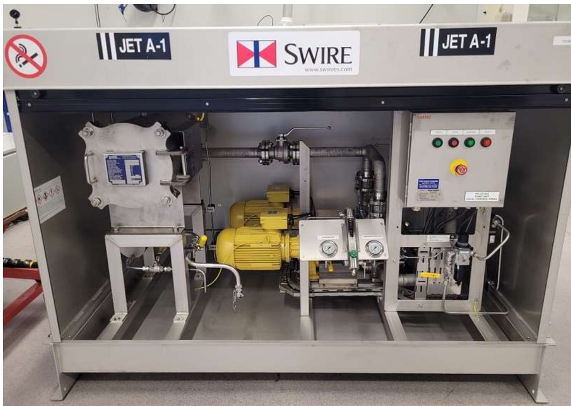
Figure 40: Helifuel Pump Unit
