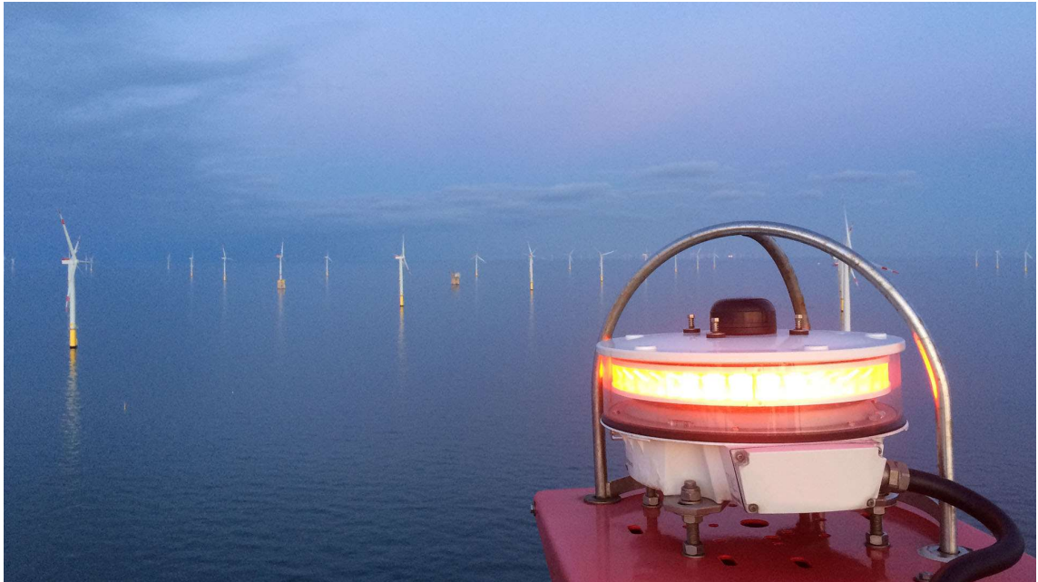
Figure 56: Obstruction light on a wind turbine
