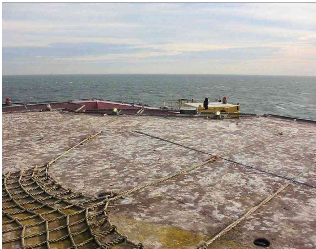
Figure 77: Guano on a helideck requires frequent cleaning.
