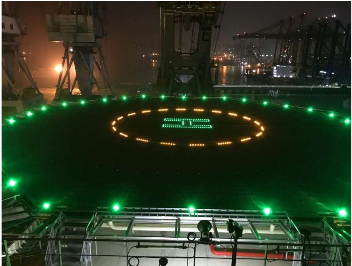
Figure 50: Circle and H Lighting at night
