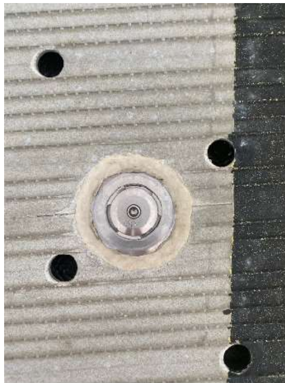
Figure 33: DIFFS Nozzle mounted into a helideck.
