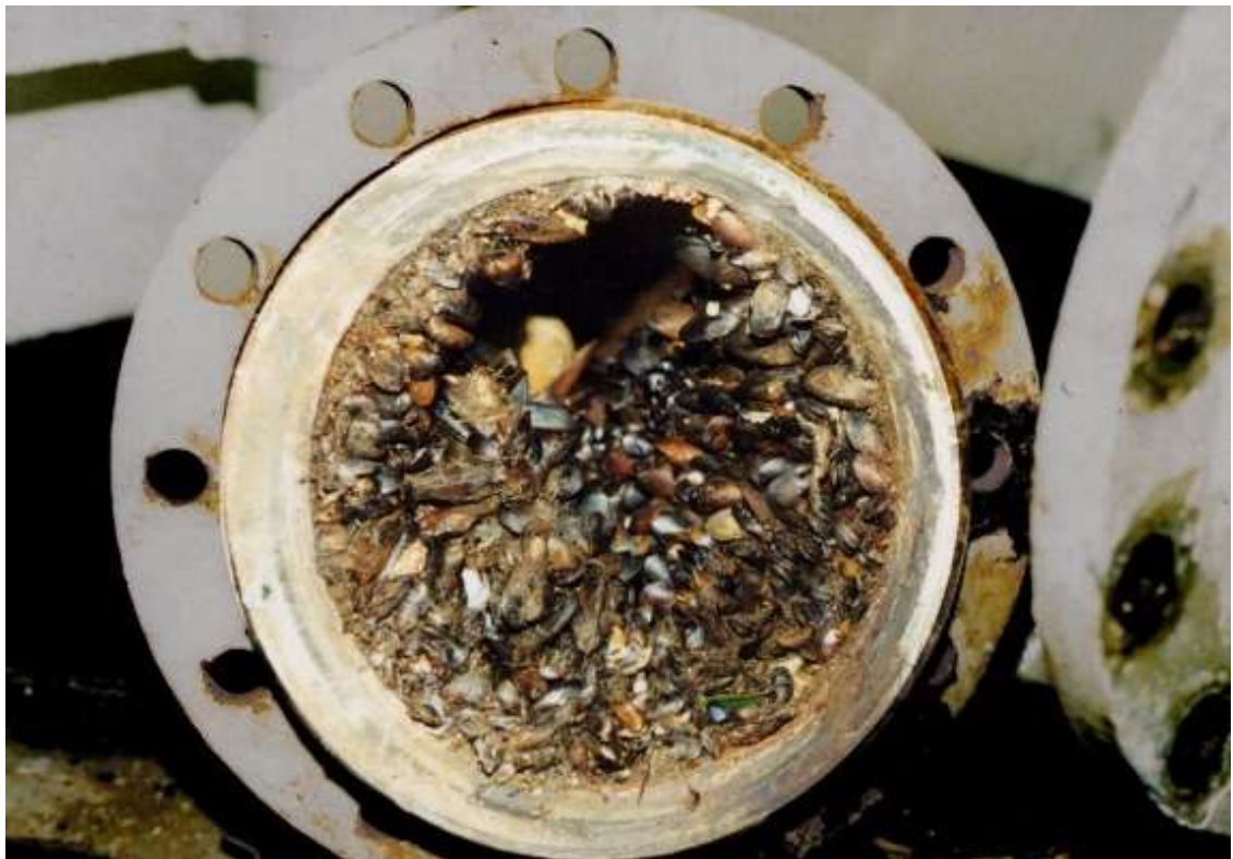
Figure 26: Marine growth within pipework
