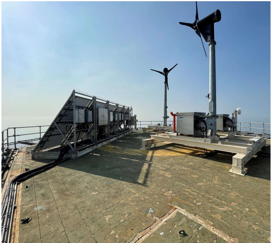
Figure 95: Helideck used for Navigational Aids/power generation.
