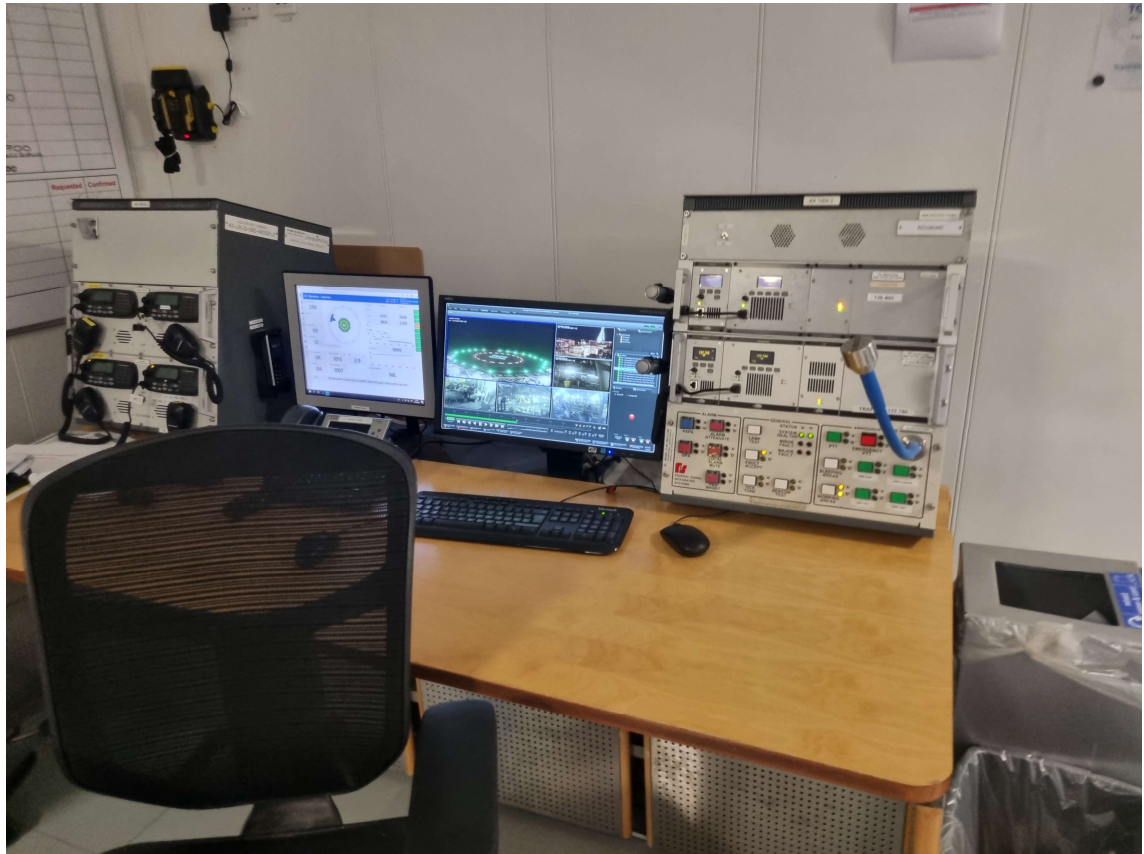
Figure 44: Radio Operator desk with CCTV, Weather Display and PAGA access
