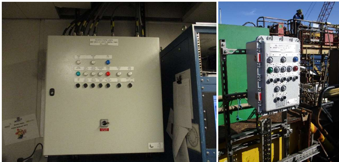
Figure 6 & 7: Safe and Hazardous Area Control panels
